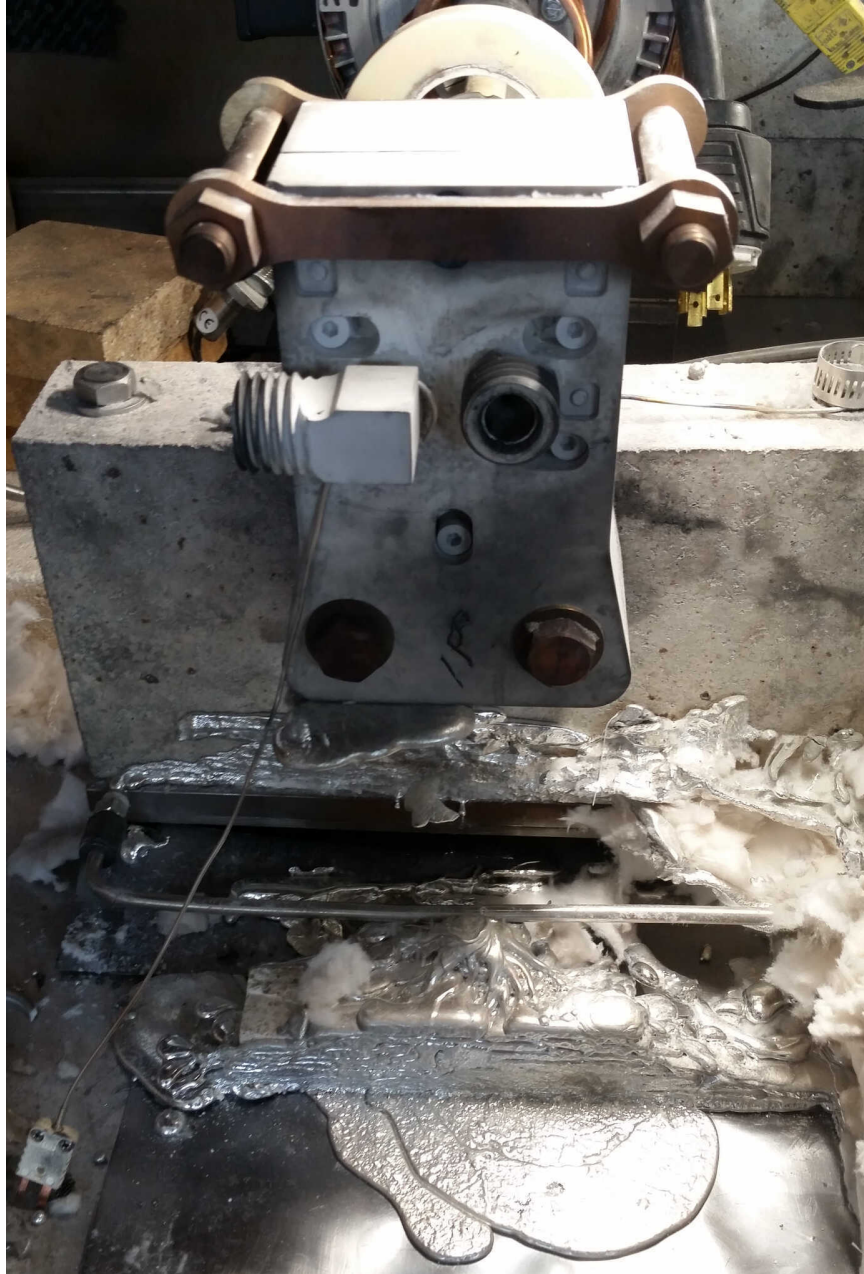
Figure 50: Leak caused by loosening of pump face seal bolts from thermal expansion
